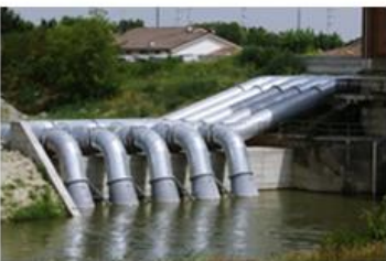
Flood control Pump stations transporting large volumes of lightly contaminated water when flooding or rainstorms occur
