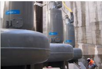
Intake station Intake station to a wastewater treatment plant
