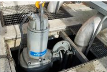
Pump stations Any pump station in the sewage collection network
