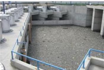
Combined Stations pumping both wastewater and storm water
